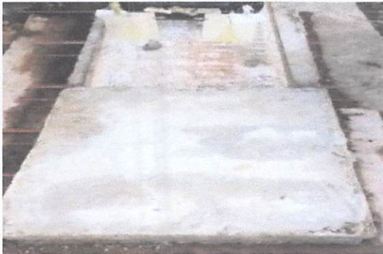
Figure 12. Concrete Slab with Void Space
