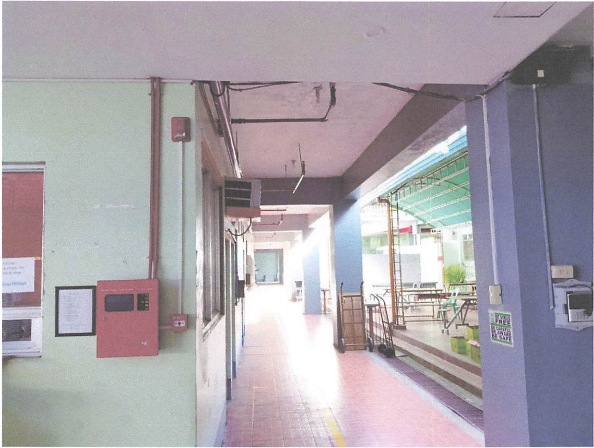
S.10. There is a central signal and fire alarm system.
