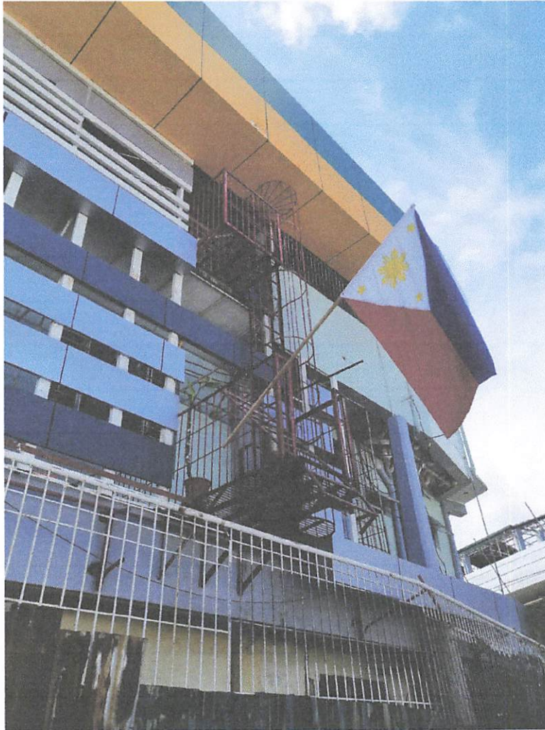
S.6. The area equipped with emergency/fire escapes which are readily accessible
