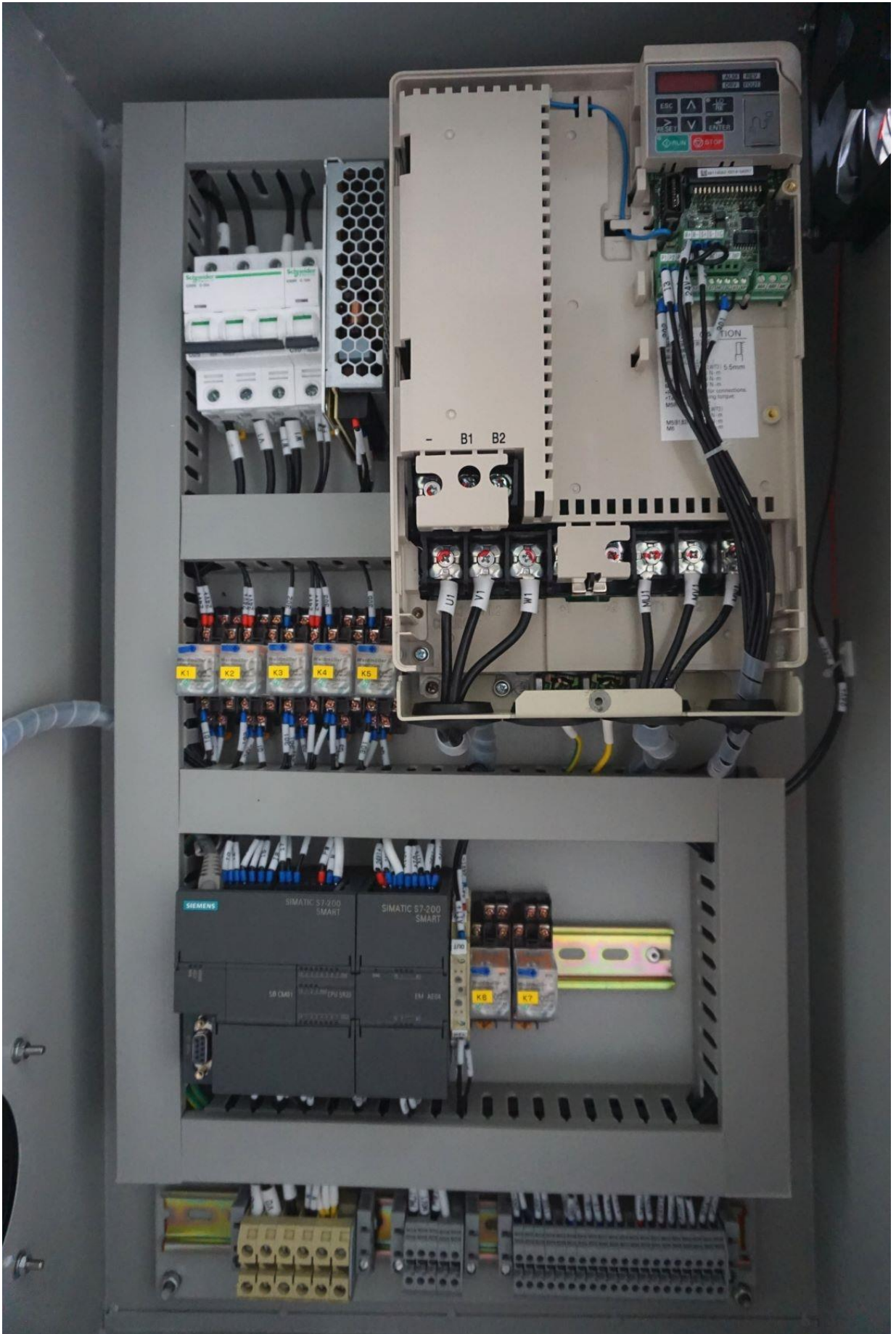
electronic control ATS
